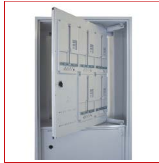
IL190290 (Messwandler 3A/42)
