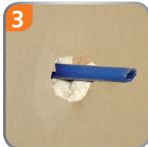
3 The drywall beats a hole with the hammer and leaves the middle spine go through, this serves as centering for the drill bit.
