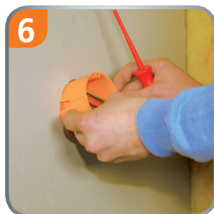
6 Without a long search of the You can use the cables Install hollow wall box.
