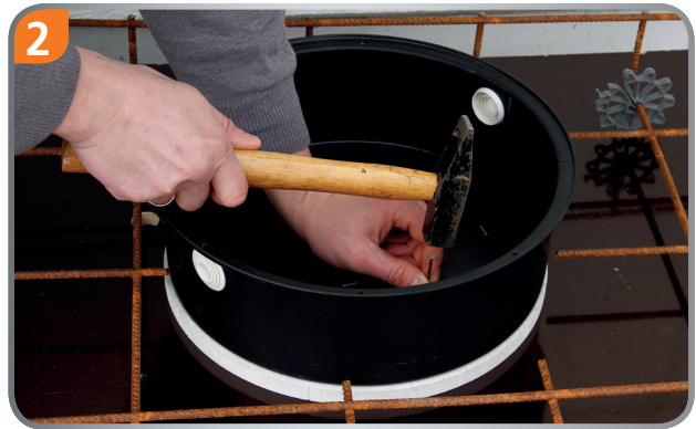
2 Nail the lightbox on the formwork (cast-in-place concrete), paste the light box on the formwork (precast factory).
